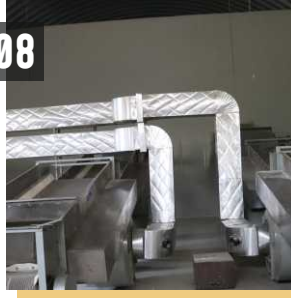
HOT DRYER SECTION
